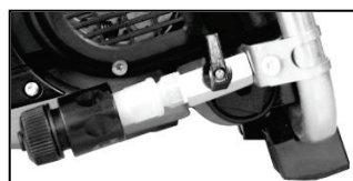
water supply closed (valve lever across)
